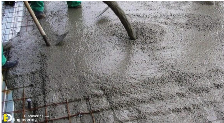
Figure 1 Typical pictorial representation of concrete as a civil Engineering material. Source [2].
